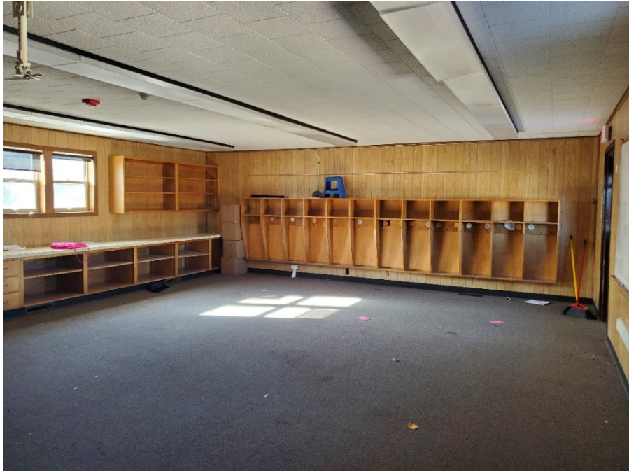
Photograph 6: Typical classroom space. No signs of water staining were noted in the ceiling finishes.
