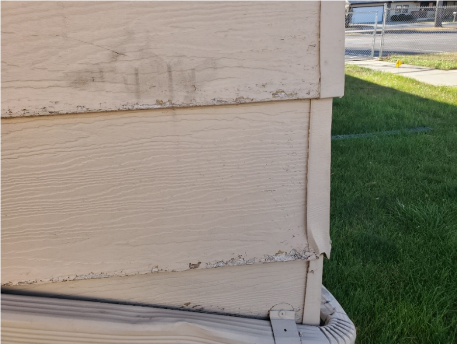
Photograph 2: Siding blemishes on Building 4. Similar siding deterioration was noted on the other units.
